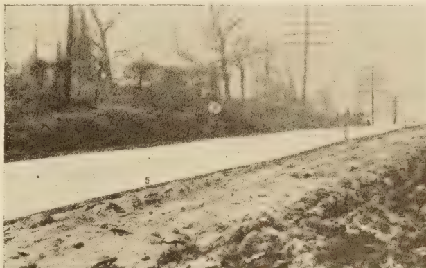
FIGURE 5.—WARPED SLABS. TRANSVERSE JOINTS ARE MARKED WITH STICKS
